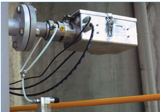
The Opsis receiver installed on the stack. The optical fibres transfer the light to the analysers for detection of gaseous compounds.
