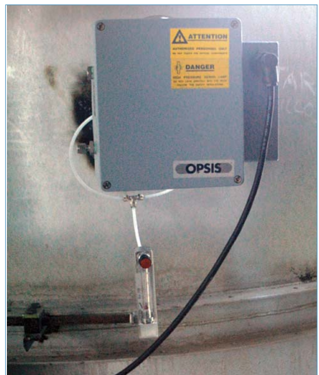
The Opsis emitter including the light source, installed on the stack.
